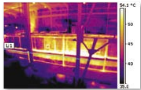
Pre-drying process viewed from machine operator's position: higher temperature due to bad extraction in the area
